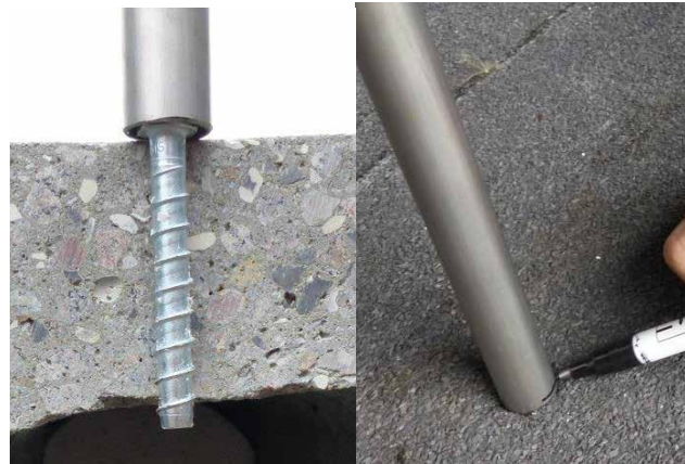
Installation with pipe support
